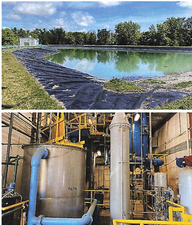
Figure 7: Melting pad (top) and treatment plant (bottom)
