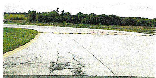
Server Pavement Distress within RW 19 RSA
