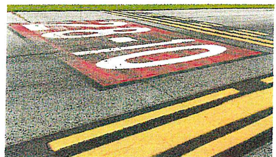
Pavement depression at RW 10-28 hold short line
