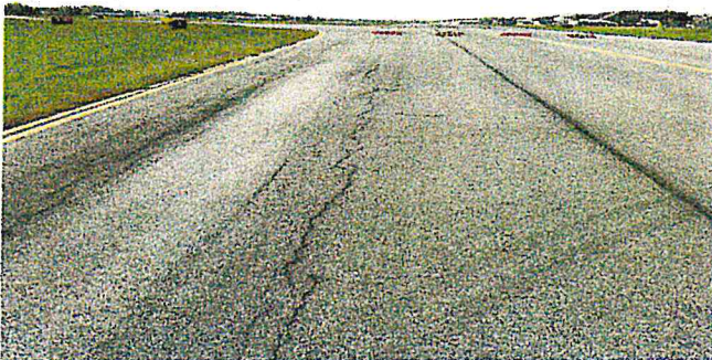
Failed pavement within paved TWA shoulder
