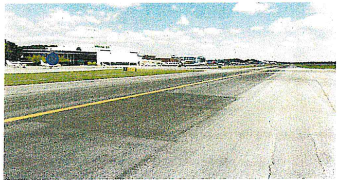
Patch of failed pavement south of TW F
