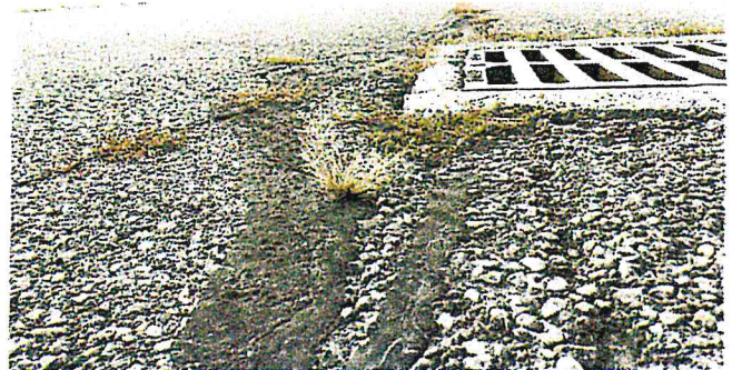
Failed pavement & drainage structure within paved TWA shoulder
