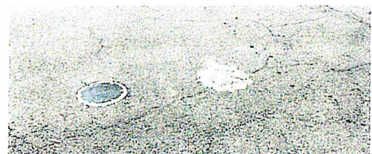
Abandoned in-pavement lights within RW 1 run-up
