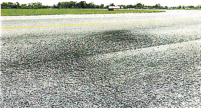
Server Pavement Distress south of TW F
