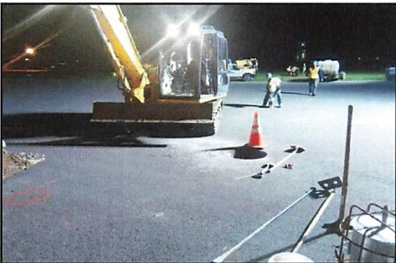
Runway 1-19 & Taxiway Edge Lighting
